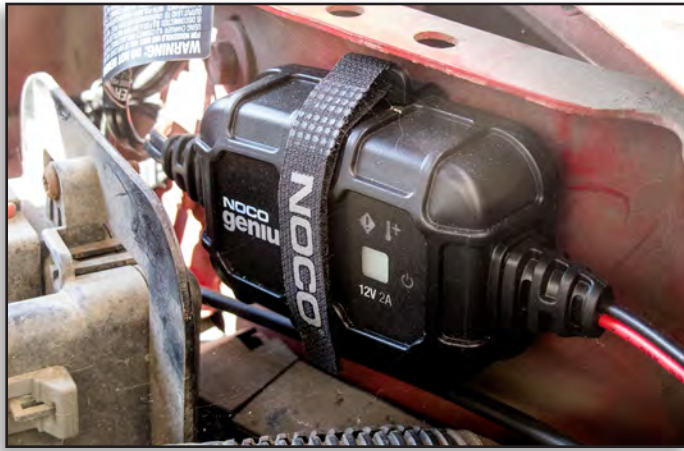
Figure 3: NOCO charger installed on fender wall.
