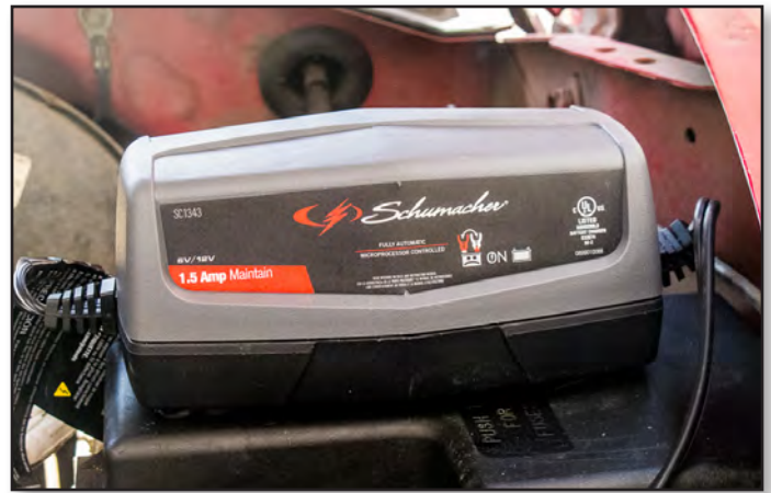
Figure 2: Schmacher trickle charger installed in engine bay.
